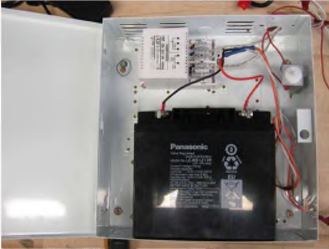
Photo 8: TRP 40/16/18 Transformer and LC-RD1217P Battery with Enclosure
